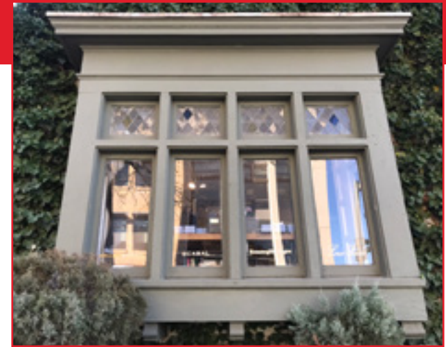
Regular maintenance such as painting exterior wood elements is a key component of historic building preservation. Central Business Historic District, City of Birmingham, photo by KDG, 2022.
