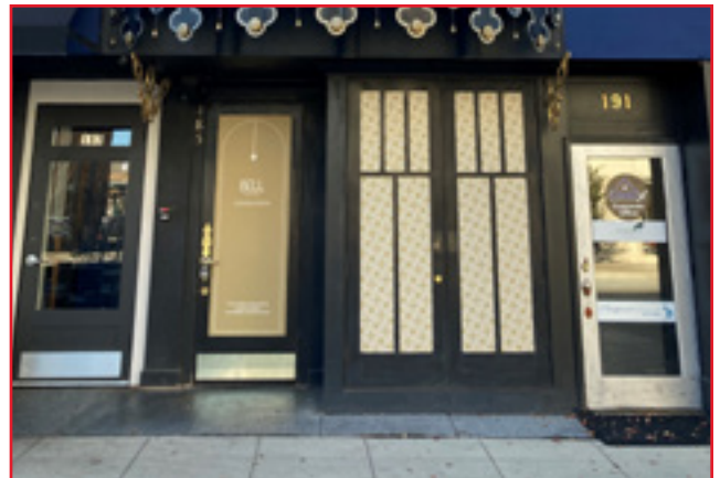
Although it is recommended that historic doors be maintained and repaired, if this cannot be done, replacement with a modern door that is complementary to the design and era of the building is acceptable. Central Business Historic District, City of Birmingham, photo by KDG, 2022.
