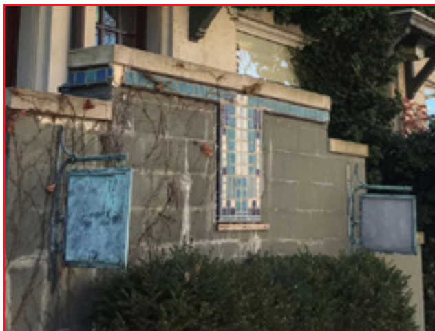
The retention of historic hanging signs on the Shain Townhouses is recommended, City of Birmingham, photo by KDG, 2022.
