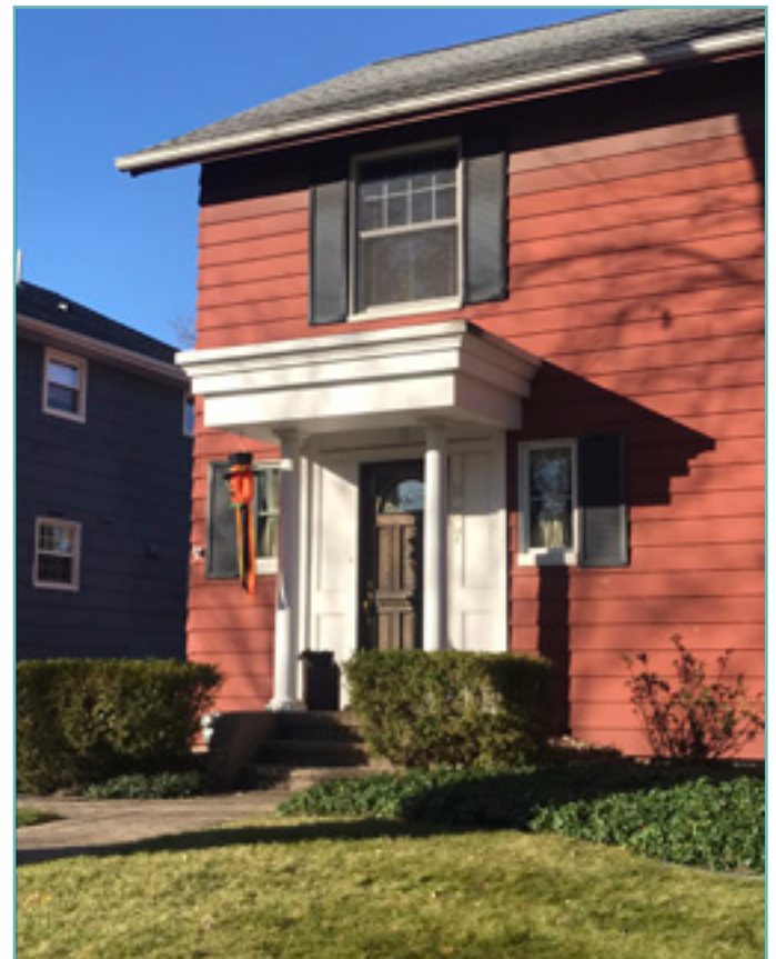
Replacement of the original porch columns is acceptable if the original columns are deteriorated beyond repair; however, it is recommended that replacement columns match the originals in terms of dimensions and detail. In the example above, the replacement columns are too slender for the porch. City of Birmingham, photo by KDG, 2022.
