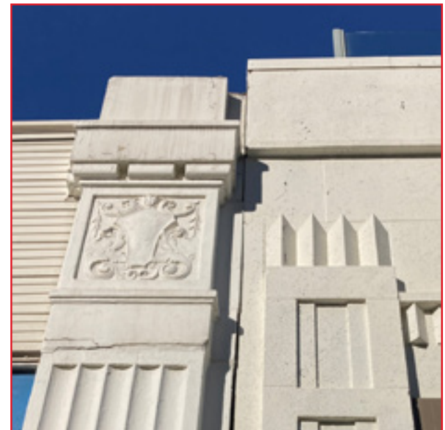
Historic exterior wall materials are often embellished with decoration and lends character to historic commercial areas. Central Business Historic District, City of Birmingham, photo by KDG, 2022.
