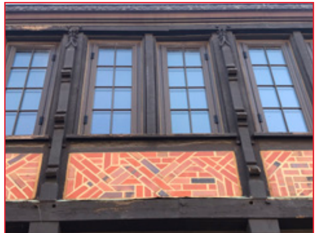
Maintenance and repair of original wood exterior details is key. The wood in the image above requires some repair from water damage and repainting. City of Birmingham, photo by KDG, 2022.
