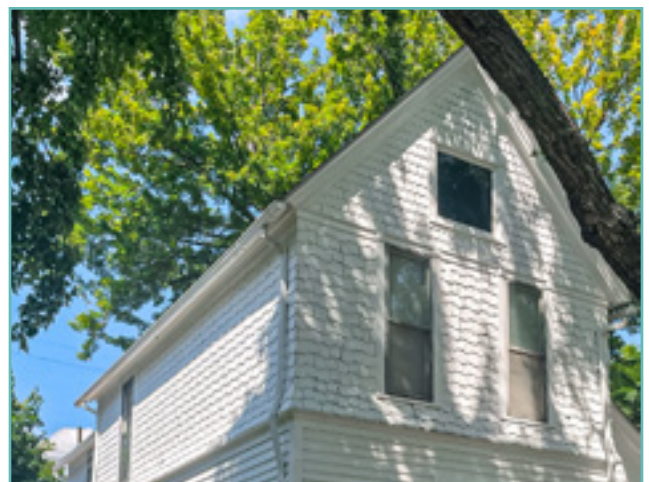
Historic wood siding and trim details create visual interest. City of Birmingham, photo by KDG, 2022.
