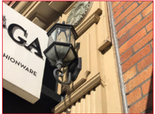
Exterior wood wall features in Birmingham's commercial district is largely limited to decorative details. City of Birmingham, photo by KDG, 2022.
