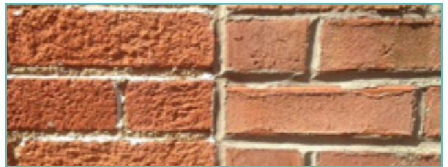
Sandblasting and other abrasive cleaning methods will severely damage historic masonry as seen here at left. The hard exterior shell of the brick, known as the fire skin, has been destroyed. This brick will begin taking on water and will deteriorate quickly. City of Birmingham, photo by KDG, 2022.
