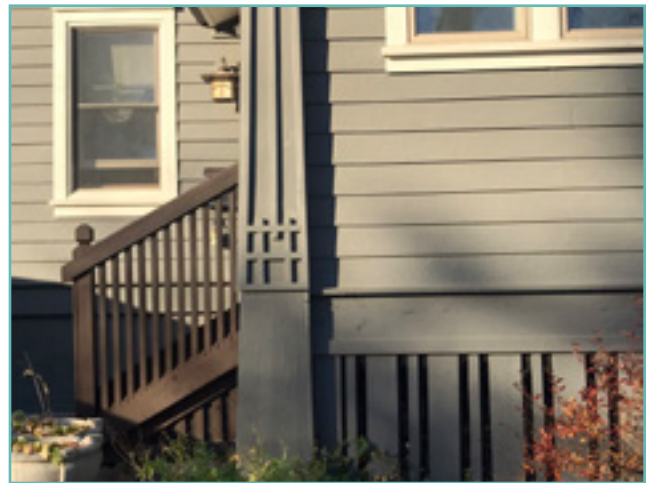
Exterior elements of this house are well maintained and by regular painting and basic maintenance. City of Birmingham, photos by KDG, 2022.
