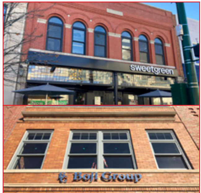
If historic windows are deteriorated beyond repair and cannot be replaced in-kind, modern replacement windows that mimic the originals are acceptable. Central Business Historic District, City of Birmingham, photo by KDG, 2022.
