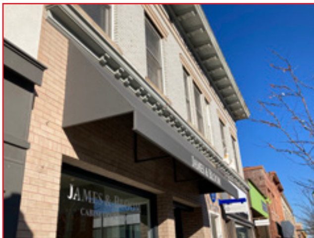
Historic awnings were generally triangularly shaped and extended outward at the base to shelter the façade. An awning may not have existed on this building historically, but this type of modern awning is acceptable. City of Birmingham, photo by KDG, 2022.
