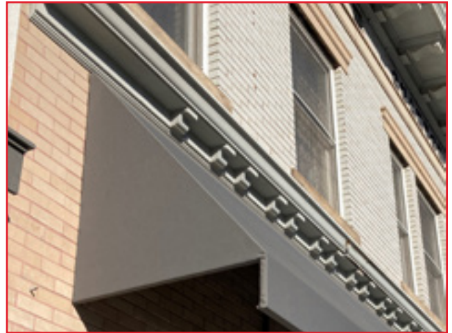
Close inspection, repeatedly completed, is key for a preventative maintenance plan. This storefront is missing modillions, likely a result of deferred maintenance, City of Birmingham, photo by KDG, 2022.
