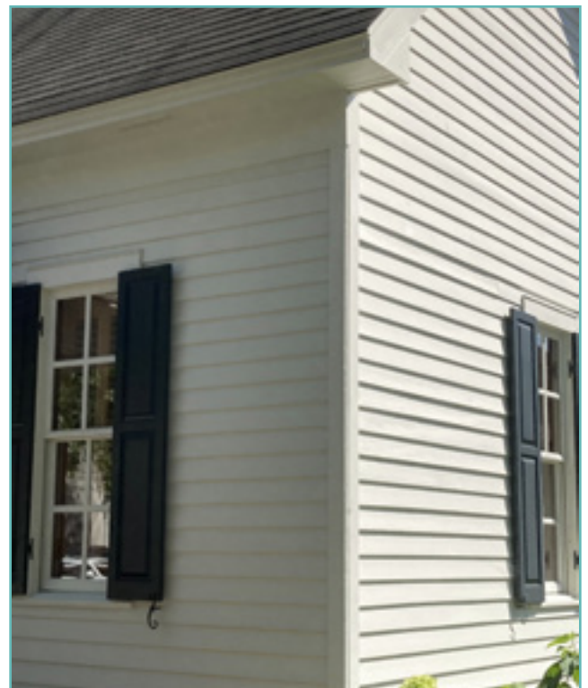
Painting helps maintain exterior wood cladding. City of Birmingham, photo by KDG, 2022.
