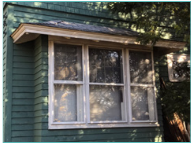
Maintaining the paint of exterior wood materials is a key component of historic house maintenance. Here, the exterior wood cladding, wood window trim wood windows, and storm windows require basic maintenance to continue functioning properly. City of Birmingham, photos by KDG, 2022.
