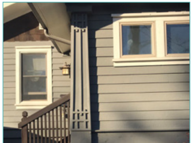
Historic wood siding and decorative exterior details. City of Birmingham, photo by KDG, 2022.
