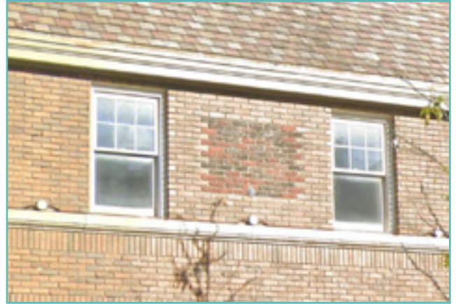
Patching historic brick with modern brick of a different color or texture on a highly visible elevation is not recommended. City of Birmingham, photo by KDG, 2022.
