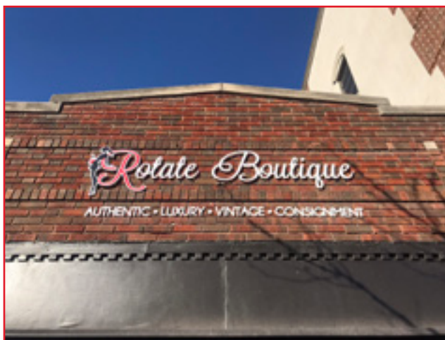
Placing signage above a designated signage band obscures the historic brick and is not recommended, City of Birmingham, photo by KDG, 2022.
