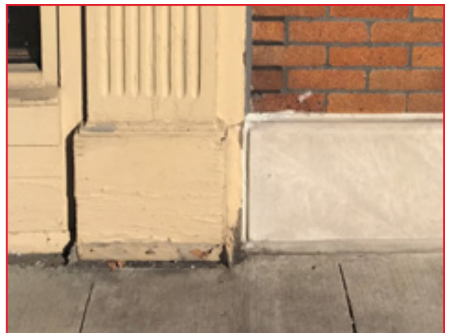
Peeling exterior paint and missing wood trim are indicative of needed maintenance, City of Birmingham, photo by KDG, 2022.
