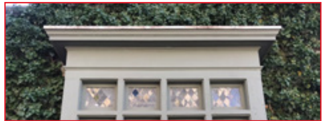
Maintaining and repairing historic windows is recommended. Where possible, the diamond pane leaded glass windows have been preserved. Central Business Historic District, City of Birmingham, photo by KDG, 2022.
