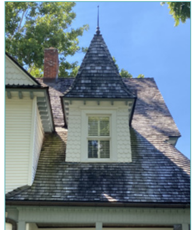
The prominent dormer and wood shingle roof are character defining features and should be preserved. Bates Street Historic District, City of Birmingham, photo by KDG, 2022.
