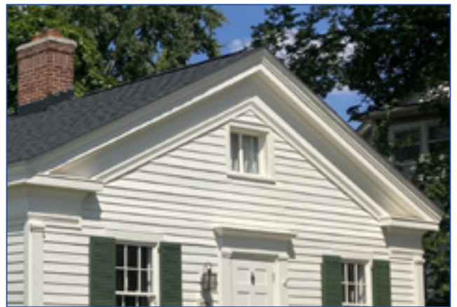
The prominent entablature and cornice returns on the gable end of the Greek Revival Hunter House. City of Birmingham, photo by KDG, 2022.
